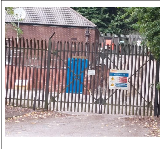
Photo 29 – Gas distribution station adjacent to southeast of Runcorn HAGI.
