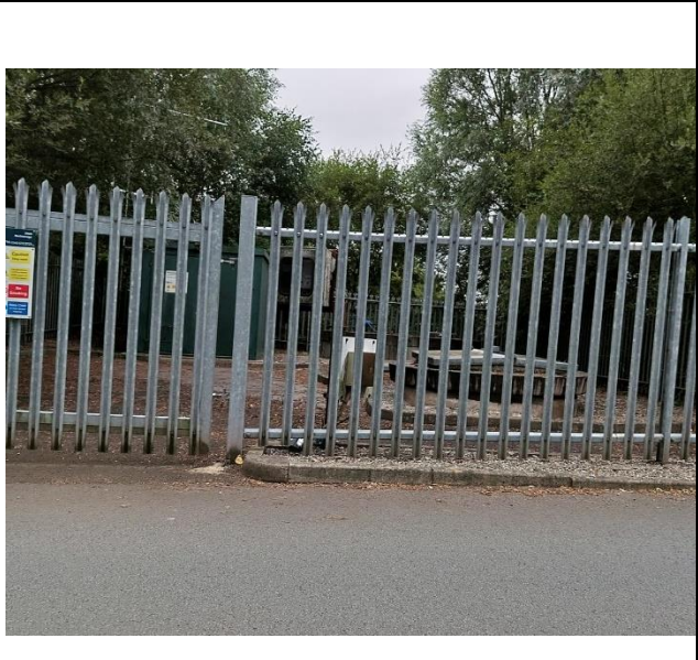
Photo 30 - Gas distribution station adjacent to southeast of Runcorn HAGI.
