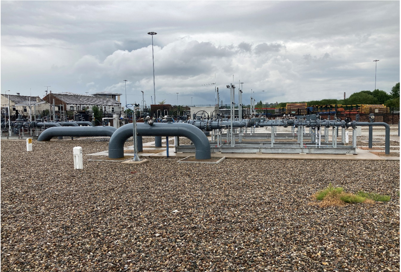
Figure NTS3.2 Photo of existing Above Ground Installation that is indicative of a HAGI
